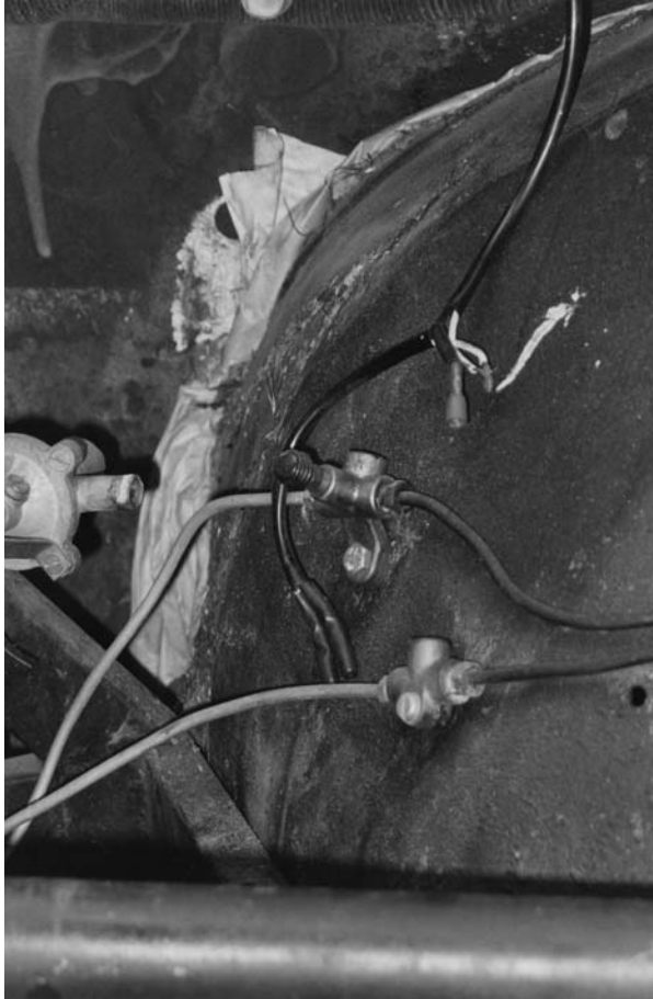
Italian newspapers and rags stuffed in the inner fender panel is a less than desirable way to add structural rigidity to a car body.
